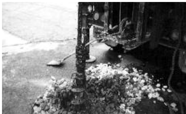
A column of muddy water rising about 2' out of the top of the augers.
