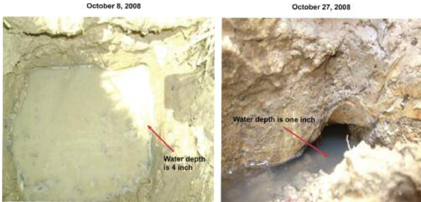
Figure 9. The void in the soil underlying the foundation at EX-3 location. Pictures are taken in October 8 and 27, 2008, respectively. Decrease in water height could be tied up to local monthly precipitation (see Figure 10). The top of the void is about 2 feet below the concrete pad. The material above the soil appears to be hardened clay or grade materials.
