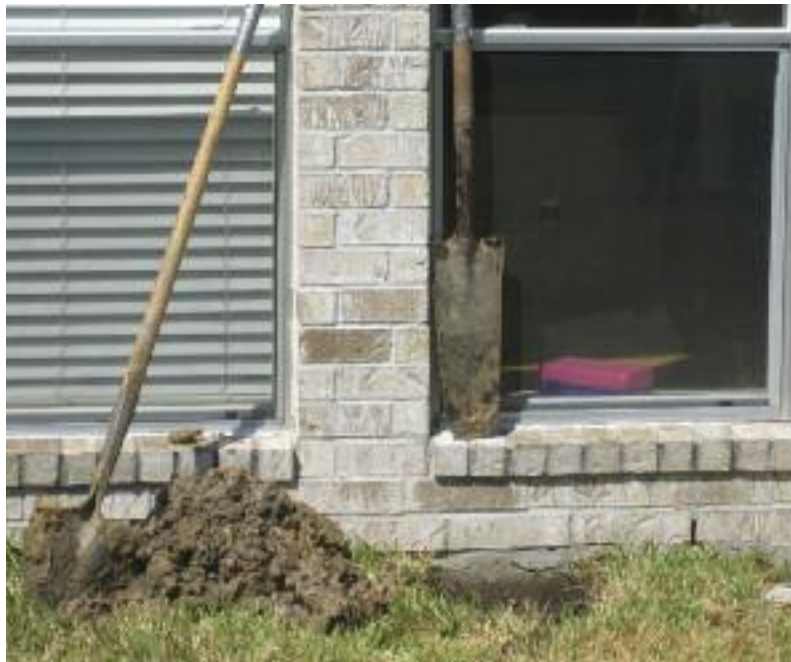
Figure 8. Picture showing the EX-3 excavation in the south wall of the foundation.
