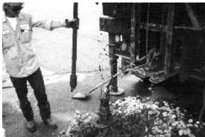
The driller holding the auger plug and rods away from the top of the augers while muddy water continues to shoot out of the augers..
