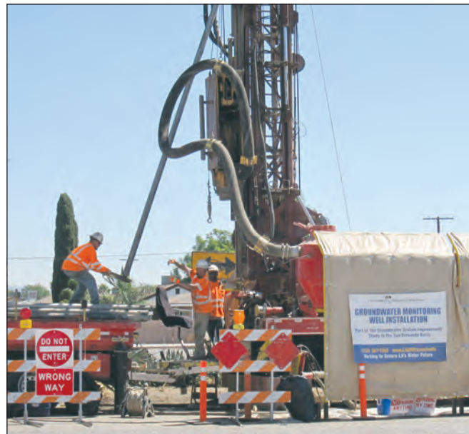
The Los Angeles Department of Water and Power (LADWP) drills exploration wells for groundwater resources in the San Fernando Valley in 2013. These wells are being used to characterize the basin’s groundwater quality. The Groundwater System Improvement Study (GSIS) will ultimately result in projects to remove contamination from the groundwater allowing the LADWP to reduce the city’s reliance on imported water providing Los Angeles with a more stable and reliable source of water. Photograph by Michael F. Forlenza, P.G.
